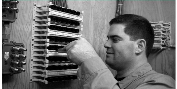
Technician Garret Miller shown wiring new West Coast Bank office at Edelweiss Village.
